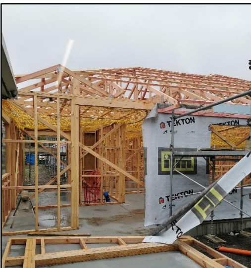
Building work is progressing on our wonderful new small home, to open next year
